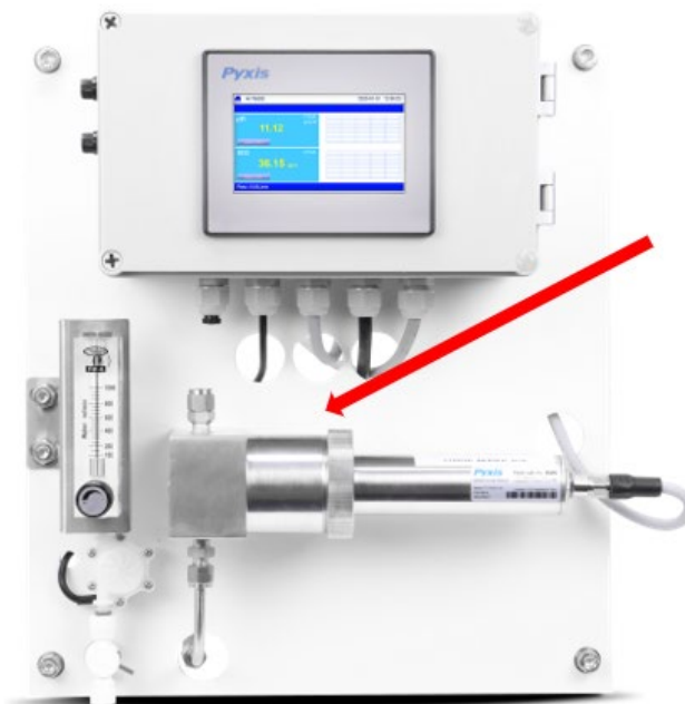
ST-007 Installed with ST-765SS-DCL Downstream of Rotameter
